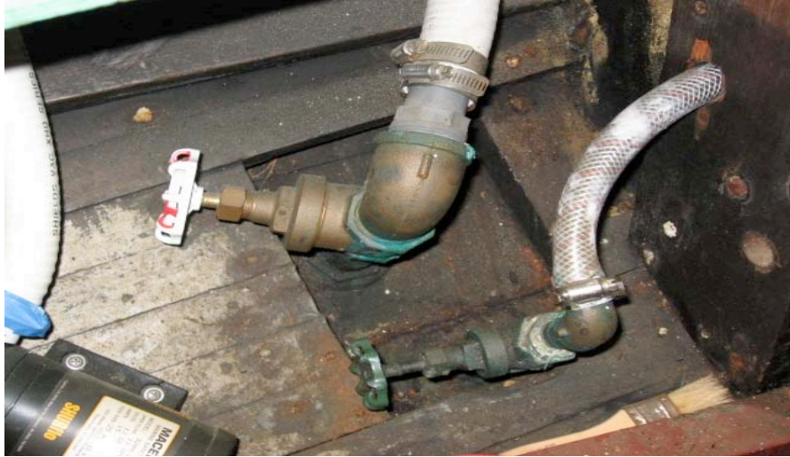
Typical thru hulls and valves
